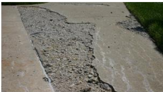
Figure 5.2 – Pavement Damage due to Freeze Thaw Cycles
